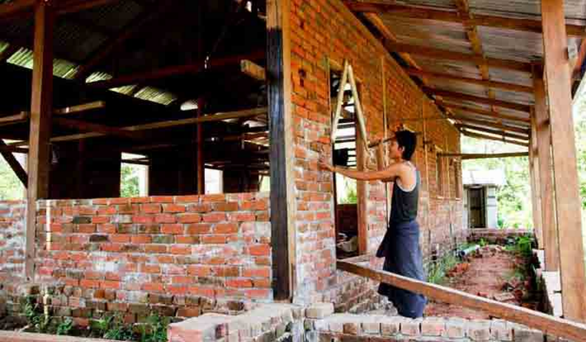
Construction of a school in an affected village. Photo by AHTF Coordinating Office
