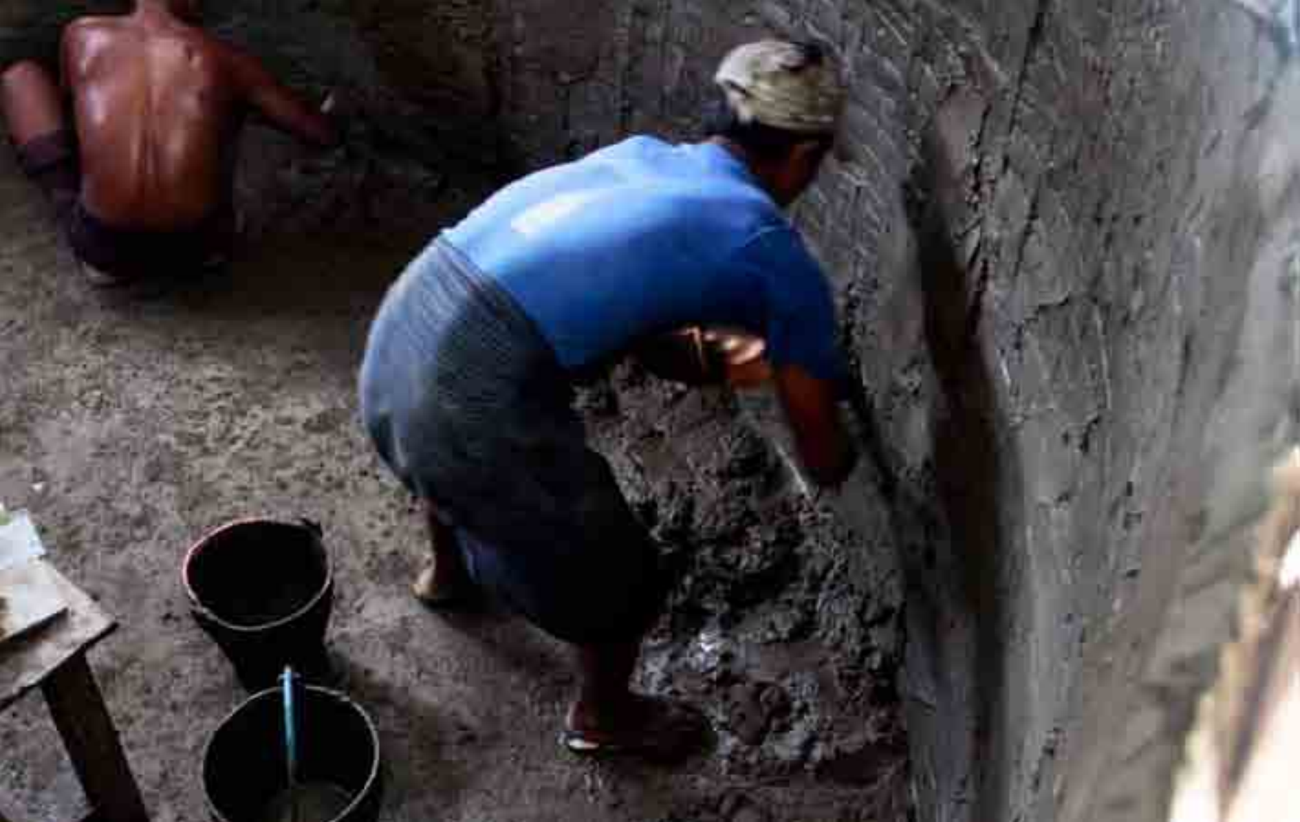
Constructing tube well as part of a water, sanitation and hygiene project by UN HABITAT in Kungyangon. Photo courtesy of UNHABITAT/Veronica Wijaya
