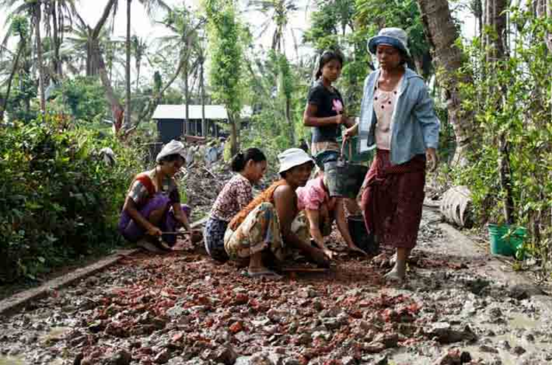
Villagers repair footpaths as part of a cash-for-work activity. Photo courtesy of UNDP
